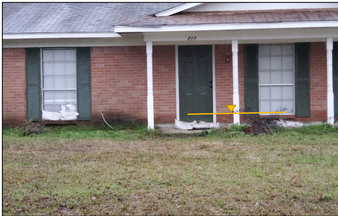
Figure 7-3. Failure of non-structural flood risk management measures during the February 2020 Flood Event. The yellow line indicates the water surface elevation during the event.
