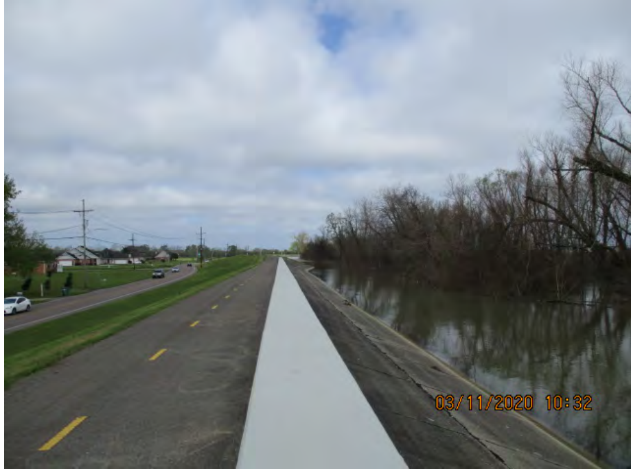
Figure 2: North facing picture near the center of the Waggaman Floodwall alignment, Jefferson Parish, Louisiana.
