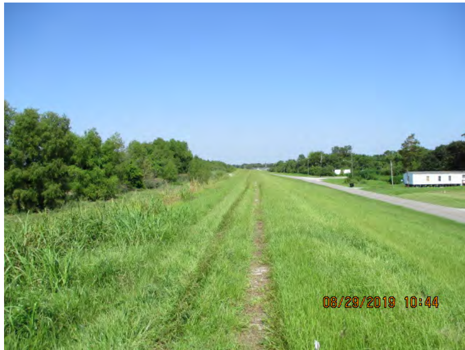
Figure 5: Northwest facing picture near the center of the alignment, Plaquemines Parish, Louisiana.
