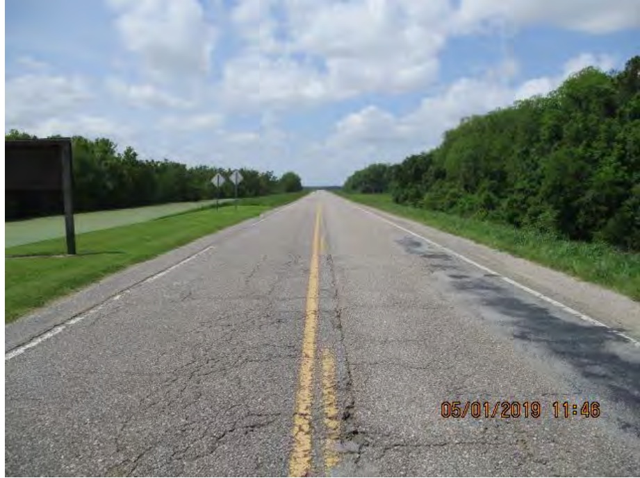
Figure 4: Southwest facing picture near the center of the alignment, Pointe Coupee Parish, Louisiana.
