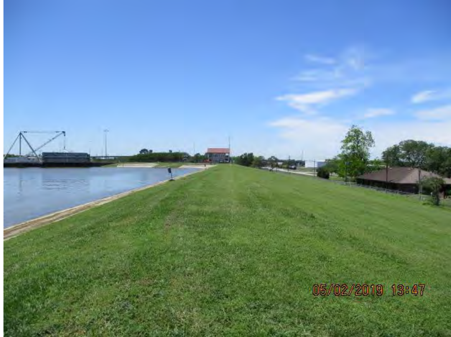
Figure 4: West facing picture near the northern end of the alignment, West Baton Rouge Parish, Louisiana.
