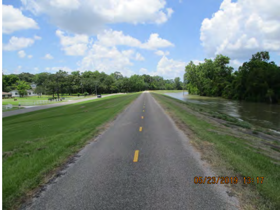
Figure 2: Northwest facing picture near the center of the alignment, Saint Charles Parish, Louisiana.
