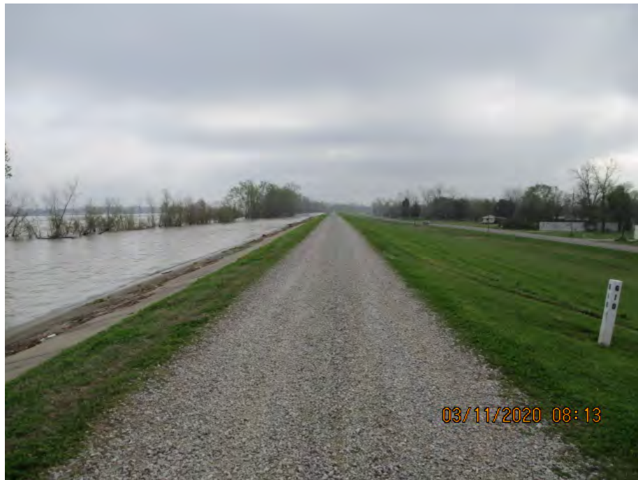
Figure 3: East facing picture near the center of the alignment, Saint James Parish, Louisiana.
