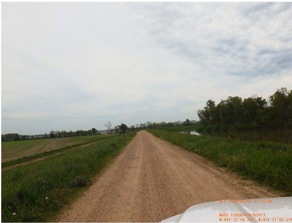
Figure 5: East facing picture from the levee crown for the proposed enlargement, Concordia Parish, Louisiana.
