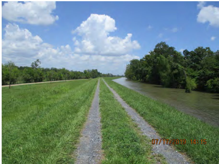
Figure 3: East facing picture near the center of the alignment, Iberville Parish, Louisiana.
