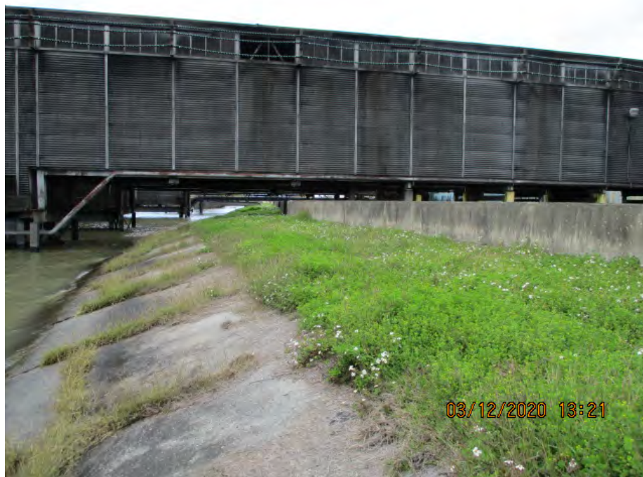
Figure 2: Northwest facing picture near the center of the alignment, St. Bernard Parish, Louisiana.
