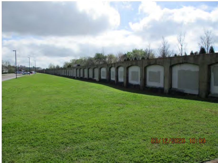
Figure 3: East facing picture near the center of the alignment, Orleans Parish, Louisiana.
