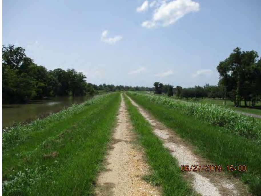
Figure 2: Northwest facing picture near the center of the alignment, Iberville Parish, Louisiana.
