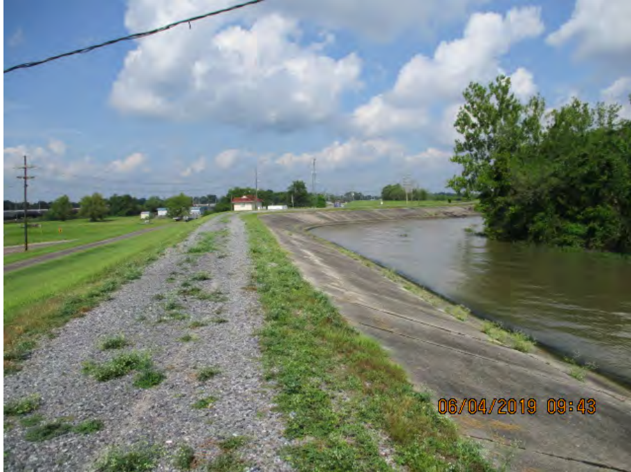
Figure 2: West facing picture near the center of the alignment, Jefferson Parish, Louisiana.
