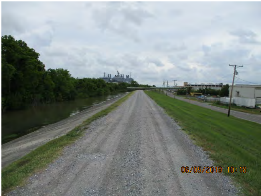
Figure 3: East facing picture near the center of the alignment, Jefferson Parish, Louisiana.
