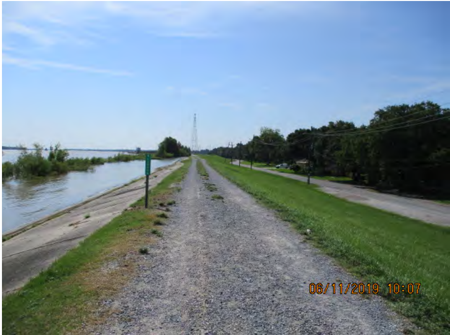
Figure 3: Southeast facing picture near the center of the alignment, Orleans Parish, Louisiana.
