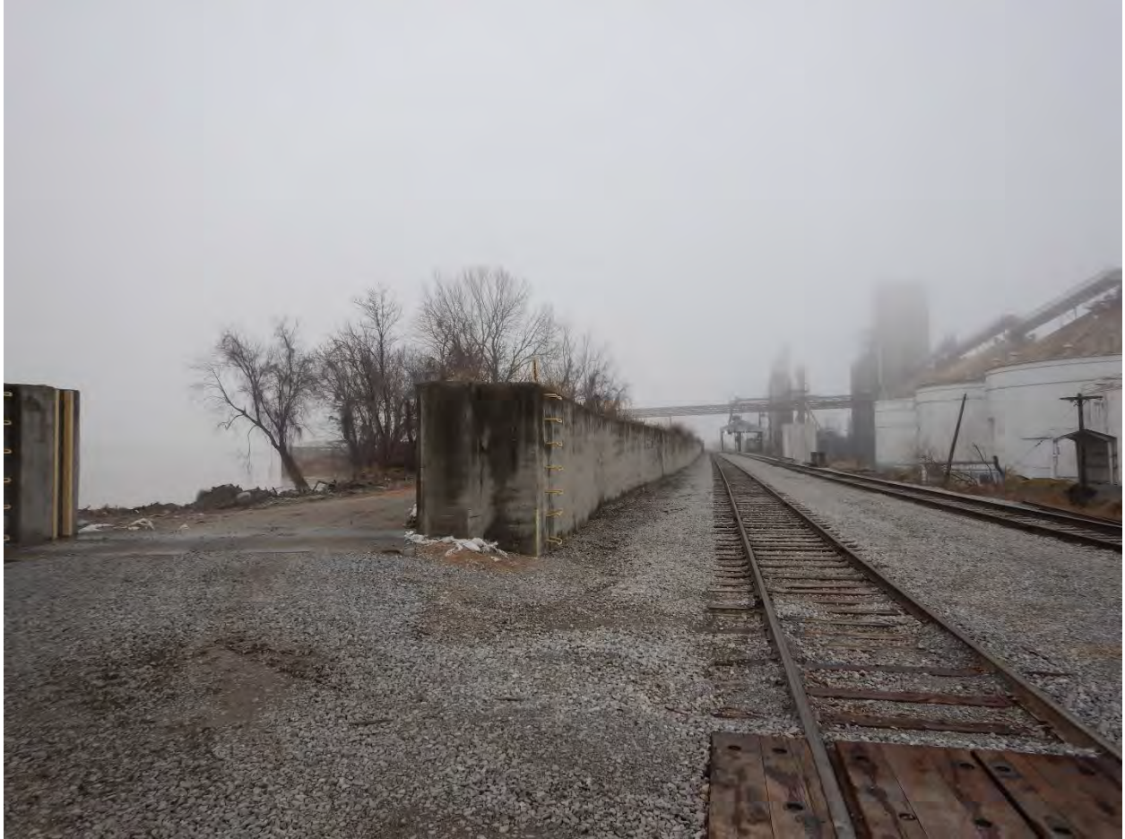
Figure 3: Photograph facing southeast (downstream) from 38 th Street along the the Cairo Floodwall near the upstream portion of the project area. Ohio River and riverside of the floodwall is shown on the left side of the photograph; landside of the floodwall and Bunge Corporation facility is shown on the right side of the photograph.
