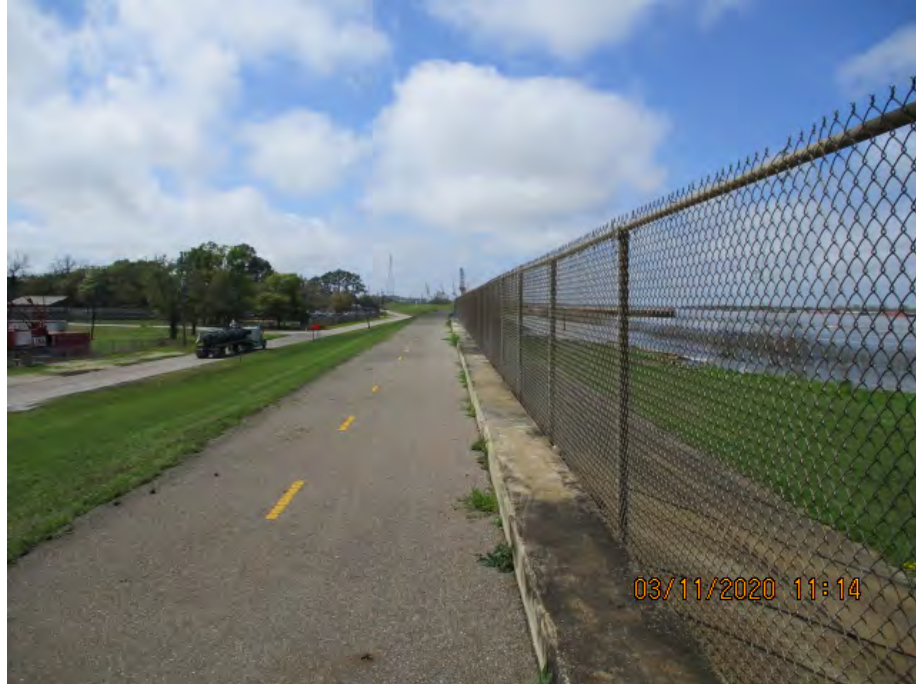
Figure 4: Southwest facing picture near the center of the Bridge City Floodwall alignment, Jefferson Parish, Louisiana
