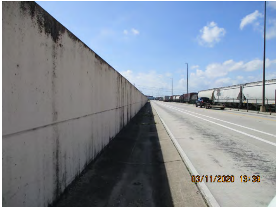
Figure 2: West facing picture near the center of the alignment, Orleans Parish, Louisiana.
