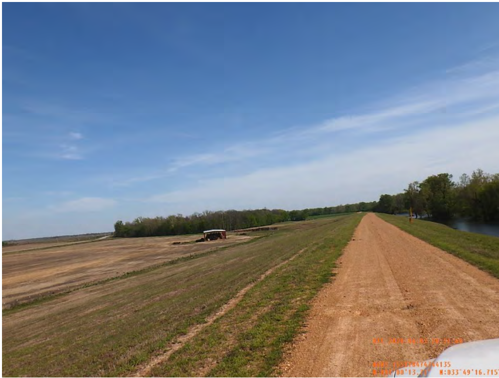
Figure 5: Southeast facing picture of the proposed seepage berm location, Bolivar County, Mississippi.
