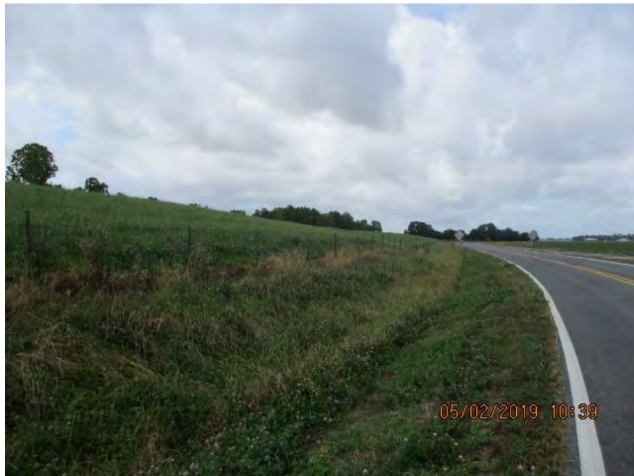
Figure 3: South facing picture near the center of the alignment, West Baton Rouge Parish, Louisiana.
