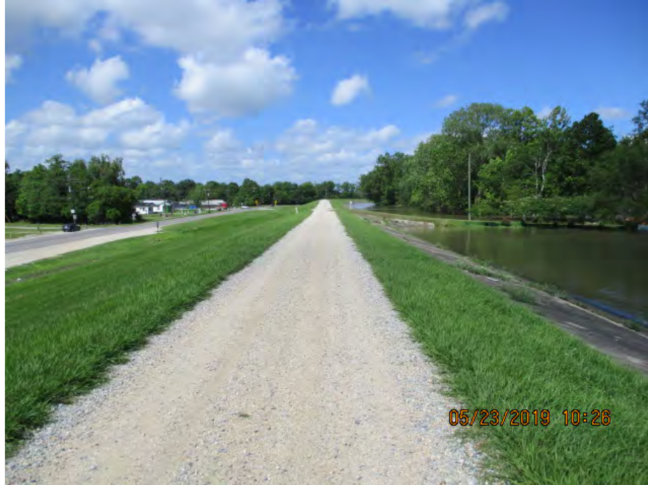
Figure 2: Southwest facing picture near the center of the alignment, Saint James Parish, Louisiana.
