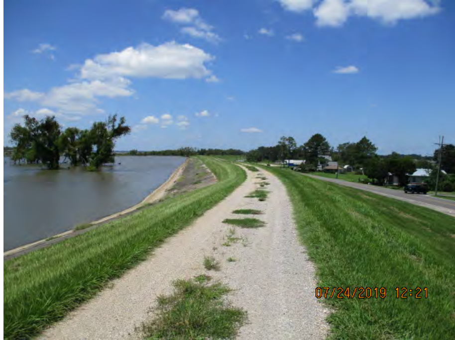
Figure 2: West facing picture near the center of the alignment, Saint James Parish, Louisiana.
