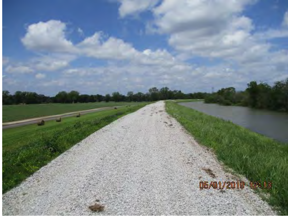
Figure 2: Northwest facing picture near the center of the alignment, Pointe Coupee Parish, Louisiana.
