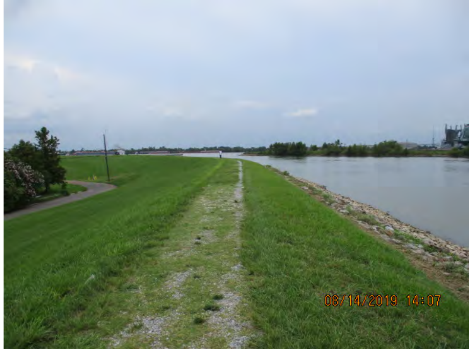
Figure 6: South facing picture near the center of the alignment on east side of IHNC Forebay, Orleans Parish, Louisiana.
