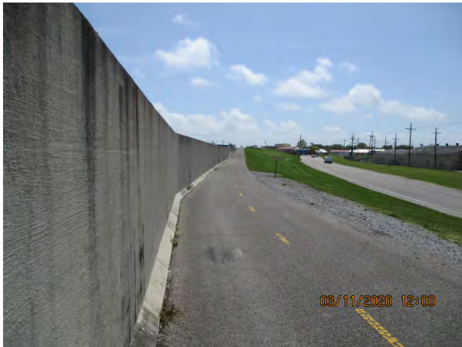
Figure 5: South facing picture near the center of Section 2 of the alignment, Jefferson Parish, Louisiana.
