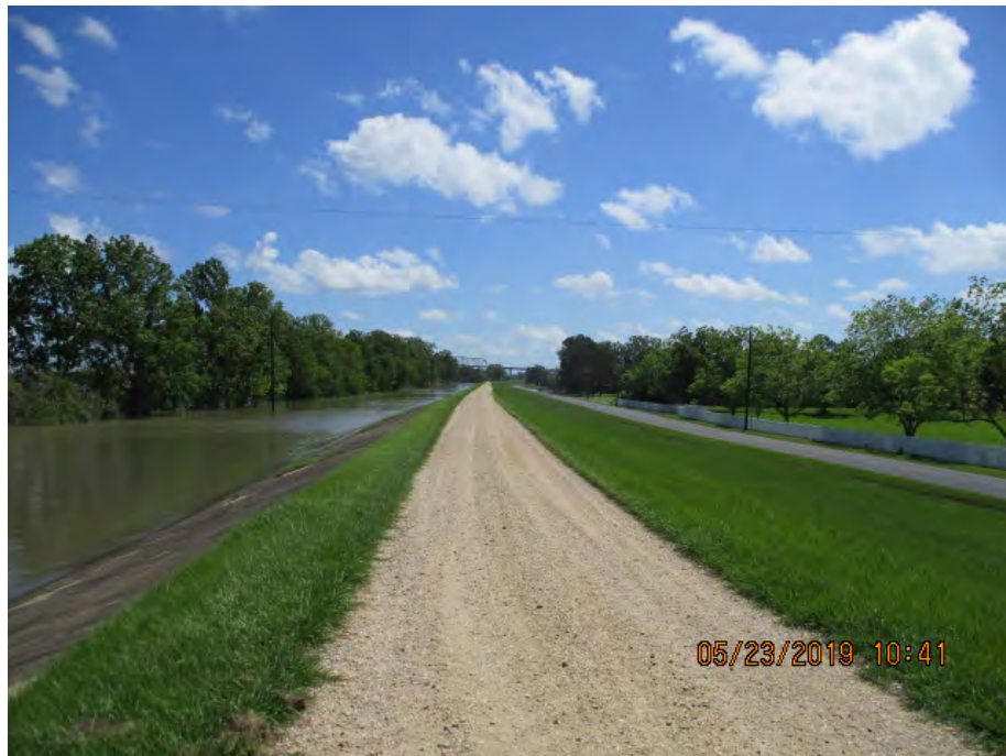
Figure 3: Northeast facing picture near the center of the alignment, Saint James and Saint John the Baptist Parishes, Louisiana.
