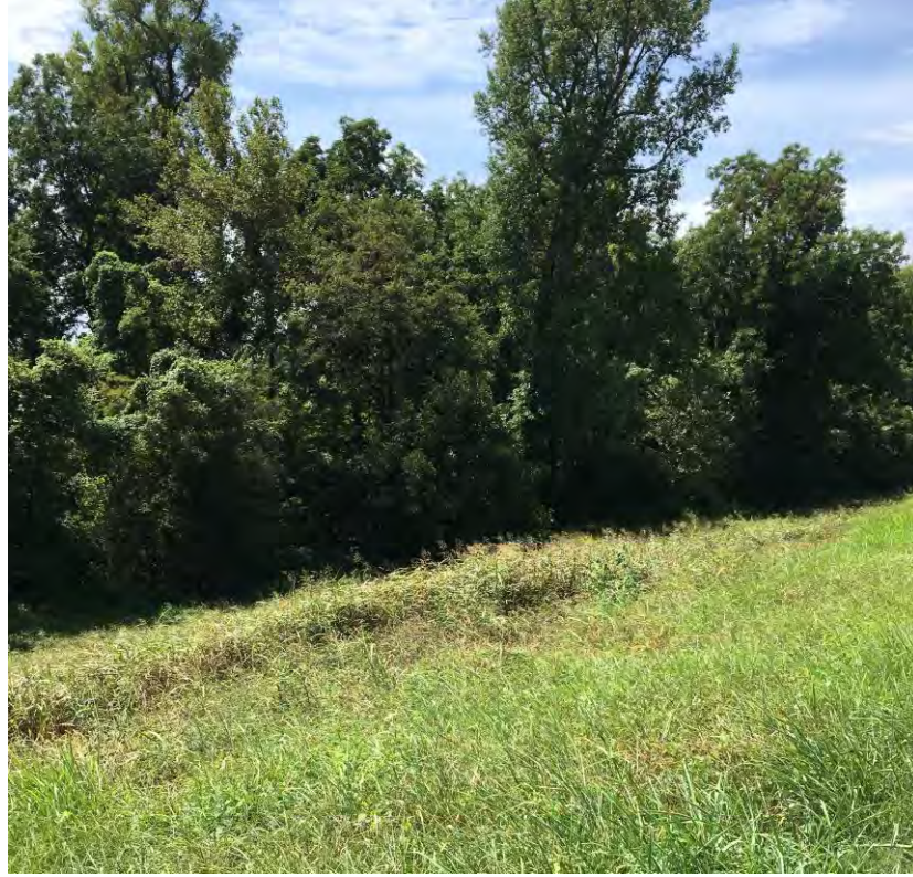
Figure 3: Photograph of scour along the riverside slope of the levee within the project area.
