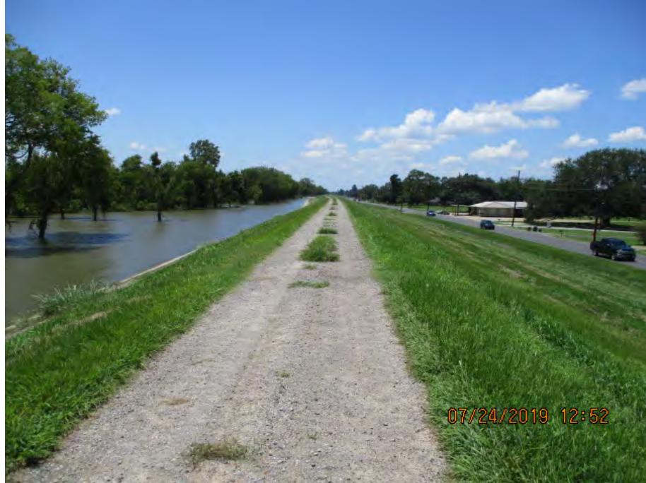
Figure 2: Southwest facing picture near the center of the alignment, Saint James Parish, Louisiana.
