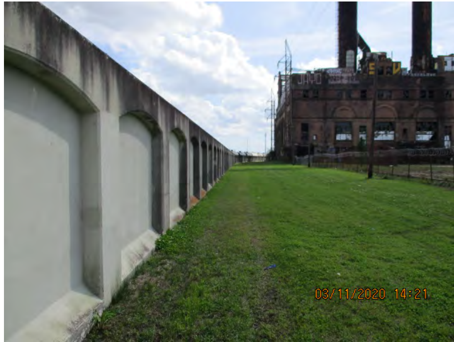
Figure 2: South facing picture near the center of the alignment, Orleans Parish, Louisiana.
