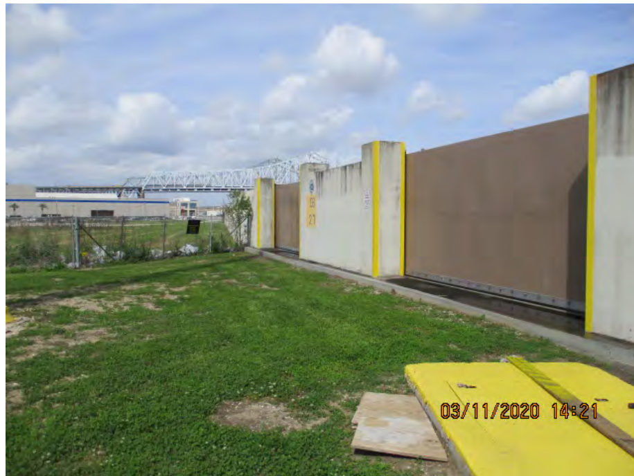
Figure 3: North facing picture near the center of the alignment, Orleans Parish, Louisiana.
