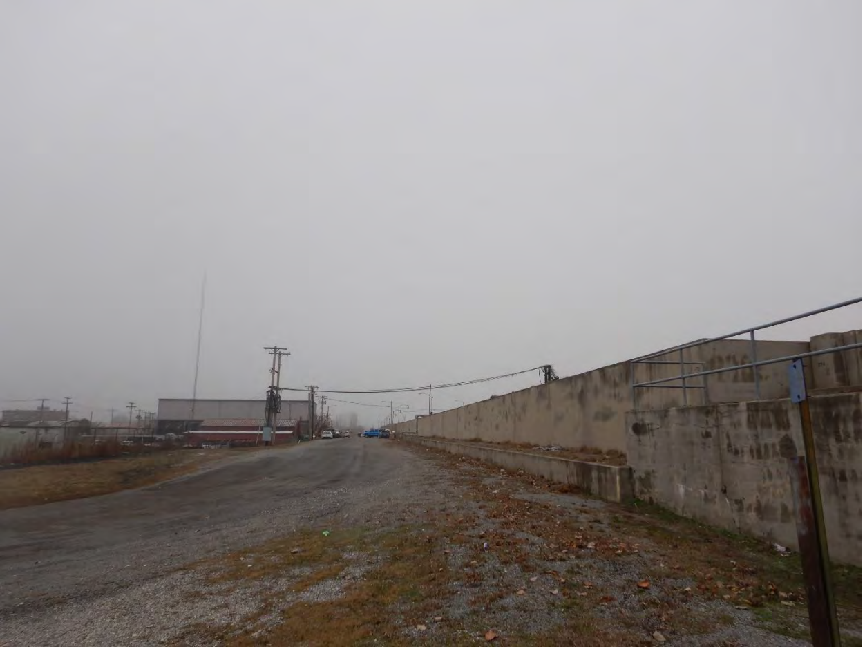
Figure 2: Photograph facing northwest (upstream) from 2 nd Street along the landside of the Cairo Floodwall near the downstream portion of the project area.
