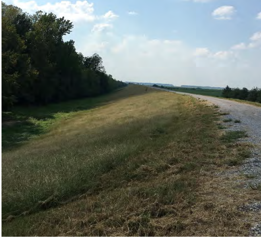
Figure 2: Representative photograph of the project area, facing downstream along the riverside levee toe within the project area.
