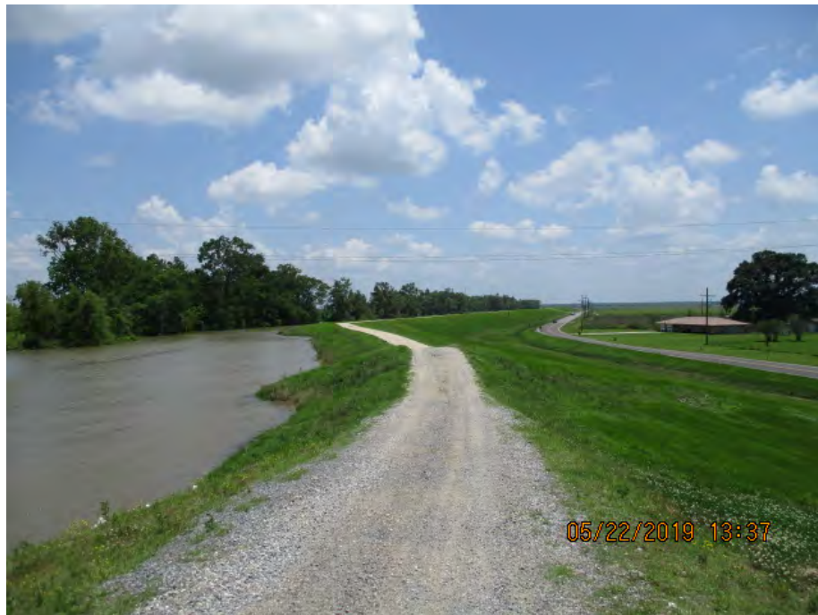
Figure 3: Southeast facing picture near the center of the alignment, Saint James Parish, Louisiana.
