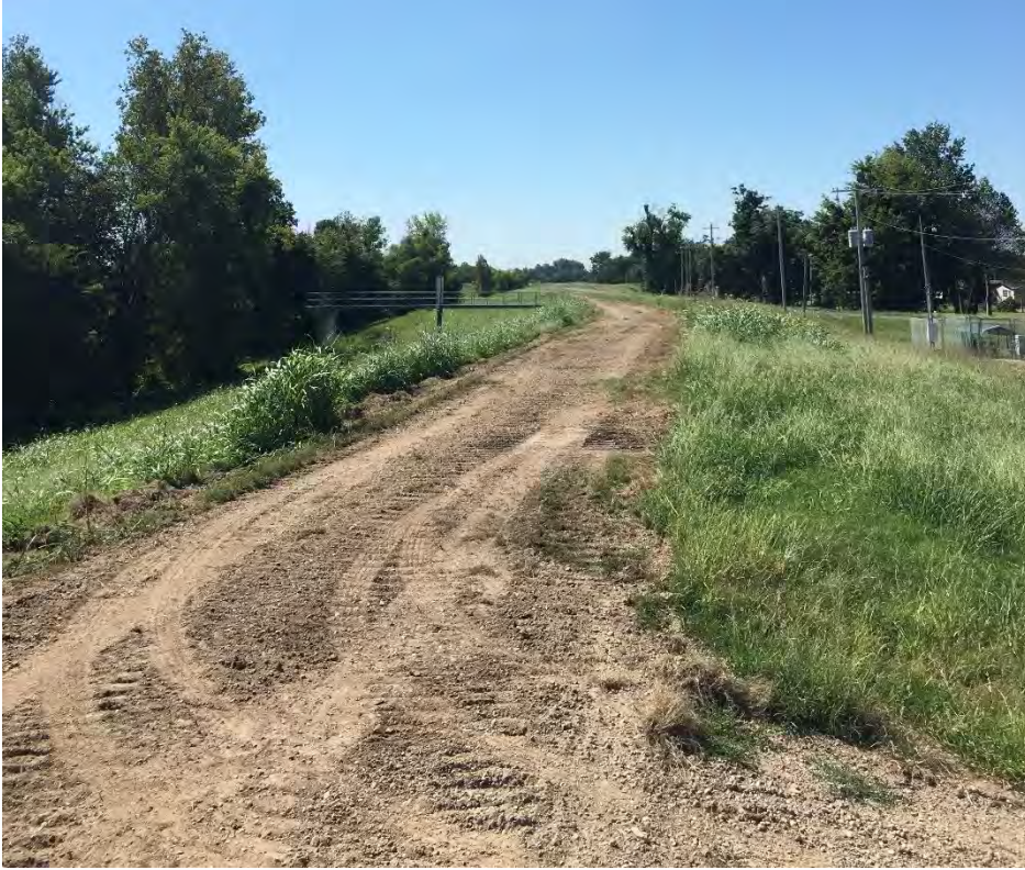
Figure 2: Representative photograph of the project area, facing downstream along the Farrenburg Levee near Missouri Highway U within the project area.
