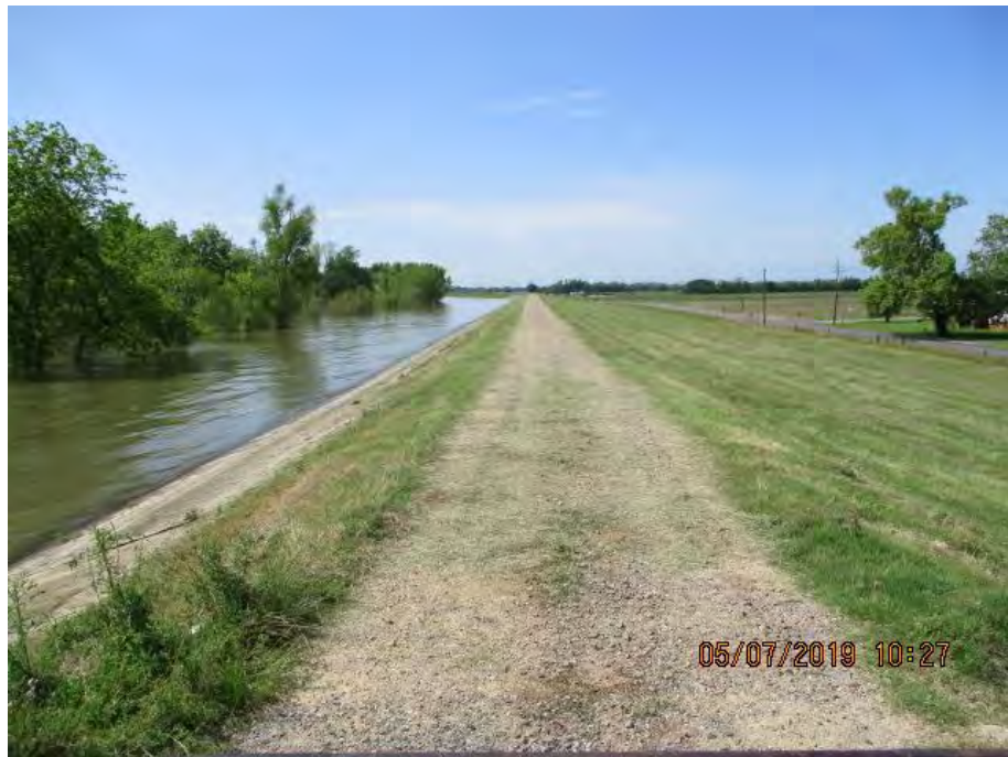
Figure 3: South facing picture near the center of the alignment, West Baton Rouge Parish, Louisiana.
