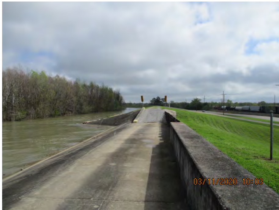
Figure 3: East facing picture near the center of the alignment, Saint Charles Parish, Louisiana.
