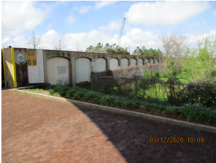
Figure 2: West facing picture near the center of the alignment, Orleans Parish, Louisiana.
