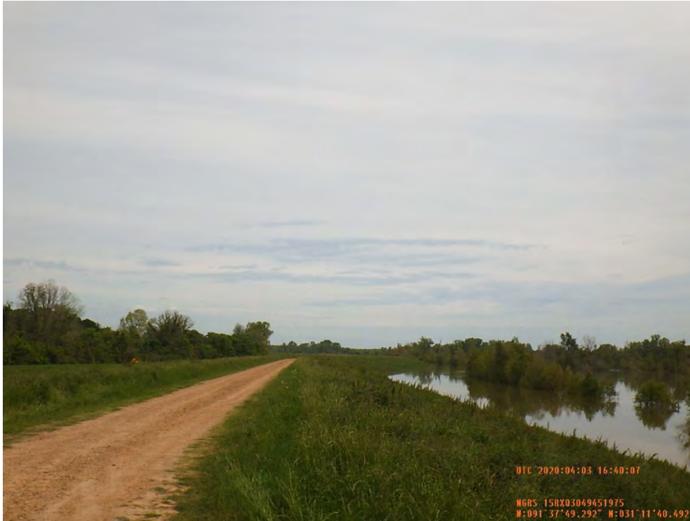
Figure 2: Northwest facing picture from the levee crown for the proposed enlargement, Concordia Parish, Louisiana.
