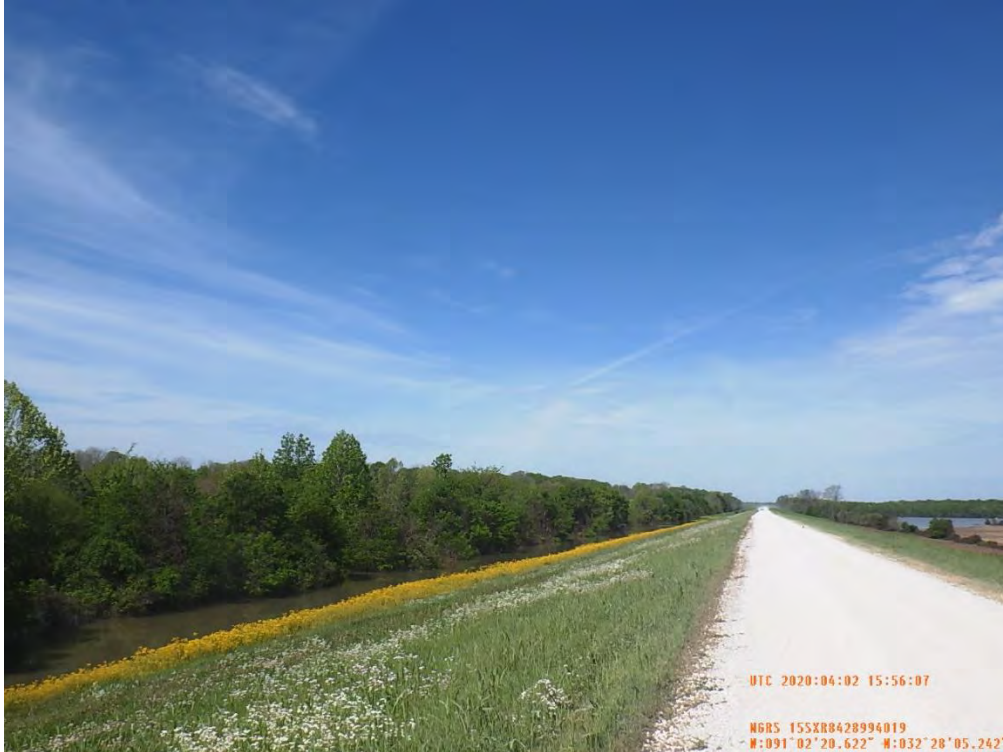
Figure 7: East facing picture of the proposed seepage berm location, Warren County, Mississippi.
