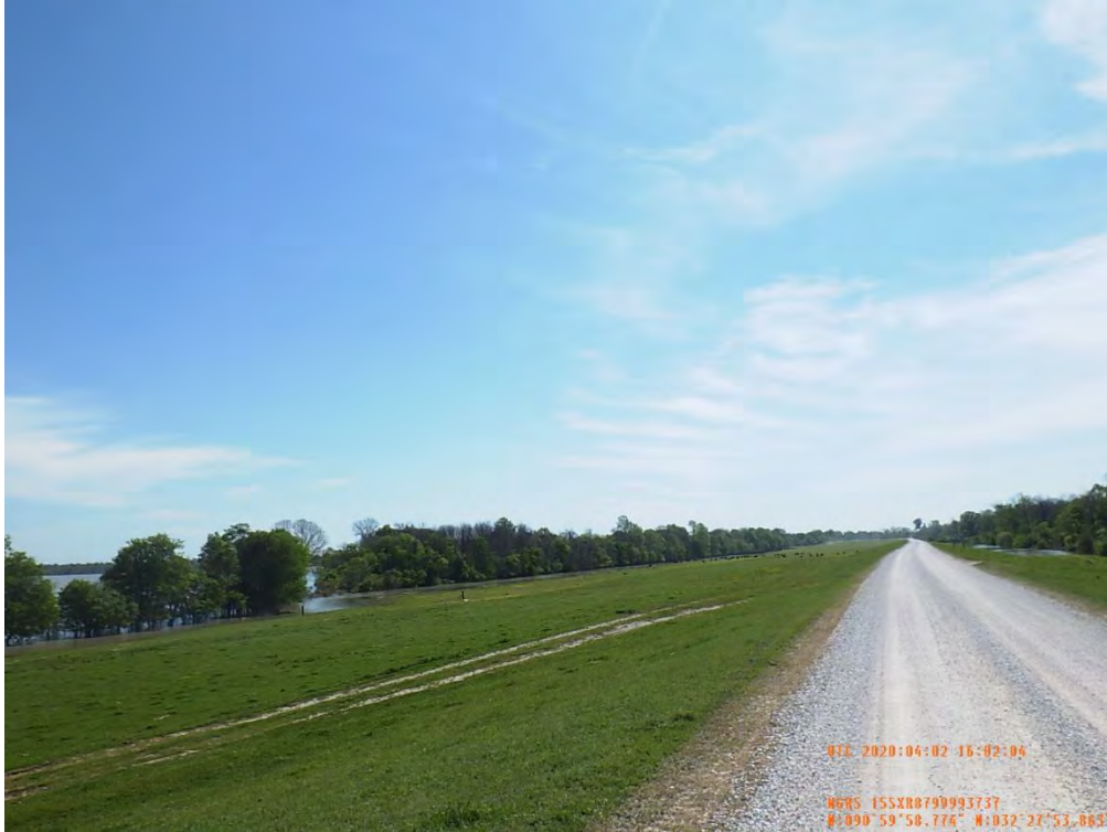
Figure 6: East facing picture of the proposed seepage berm location, Warren County, Mississippi.
