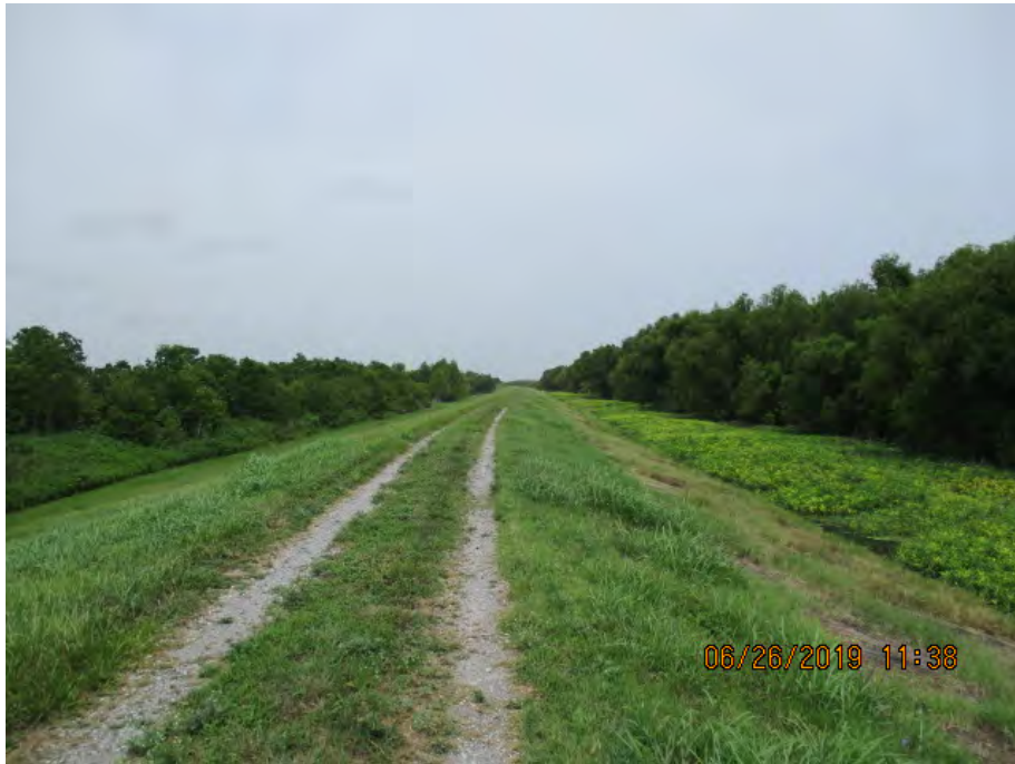
Figure 2: West facing picture near the center of the alignment, Plaquemines Parish, Louisiana.
