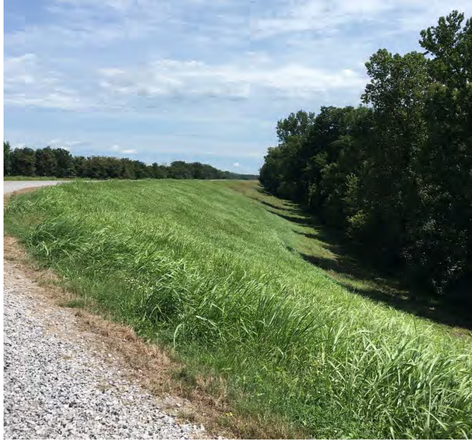
Figure 2: Representative photograph of the project area, facing the riverside levee toe within the project area.
