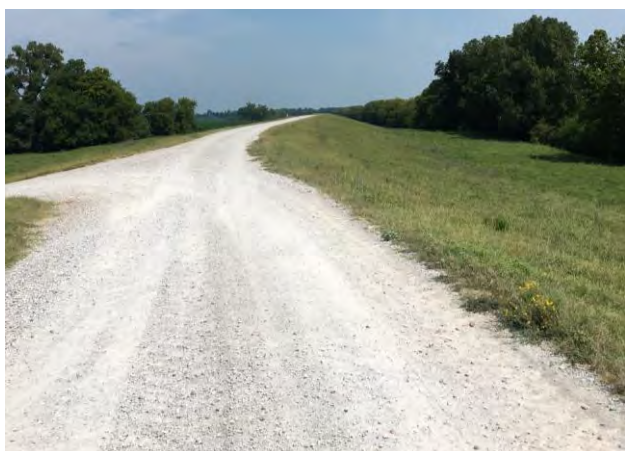
Figure 2: Facing NW (upstream) along the mainline Mississippi River Levee crown within the proposed project boundaries.
