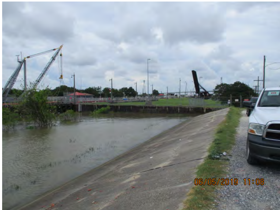
Figure 5: South facing picture near the center of the alignment, West side of the Harvey Canal, Jefferson Parish, Louisiana.
